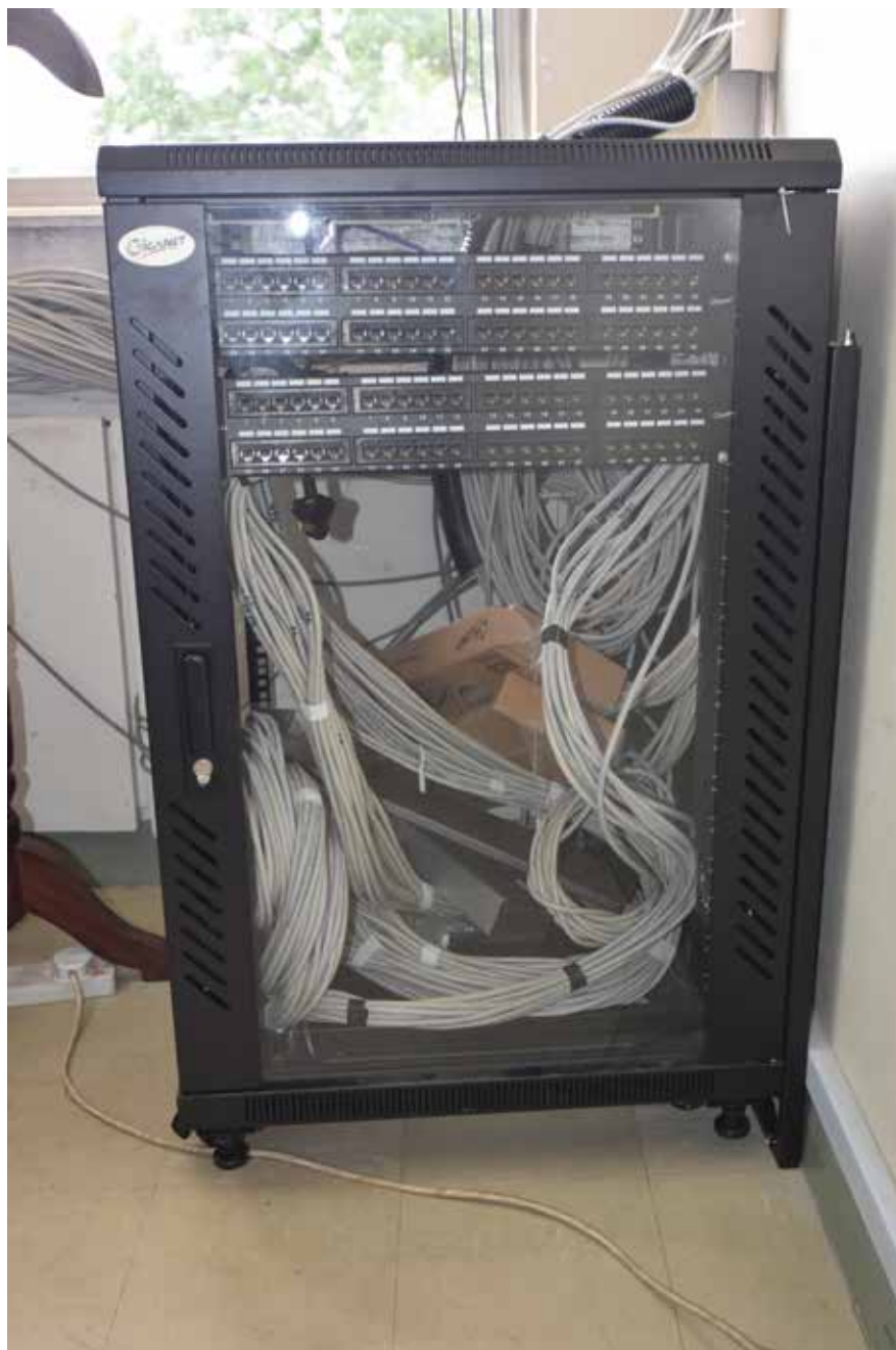
A rack cabinet for network switches installed in one of the offices at KLB.
